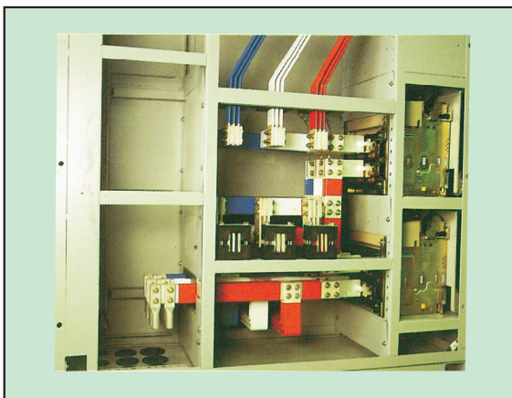
ACB Zone、Busbar Zone and Cable Zone
